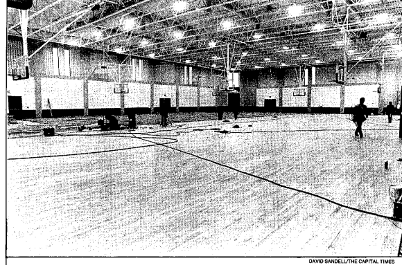
New fieldhouse Work continues into the just-started school year on the new $3 million fieldhouse at Memorial High School. The fieldhouse, which has been under construction since July 1991, is targeted for completion Sept. 18.
