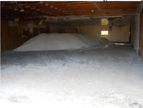
Salt in loading dock area
