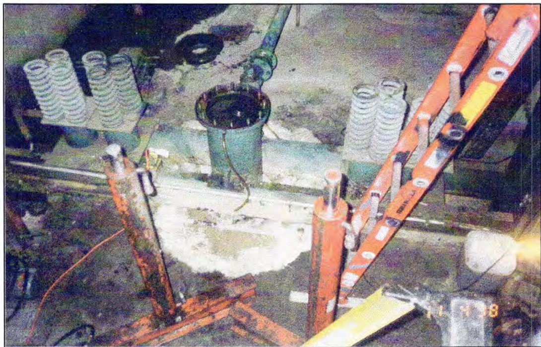
Photograph 2 Hydraulic cylinder at base of freight elevator room.
