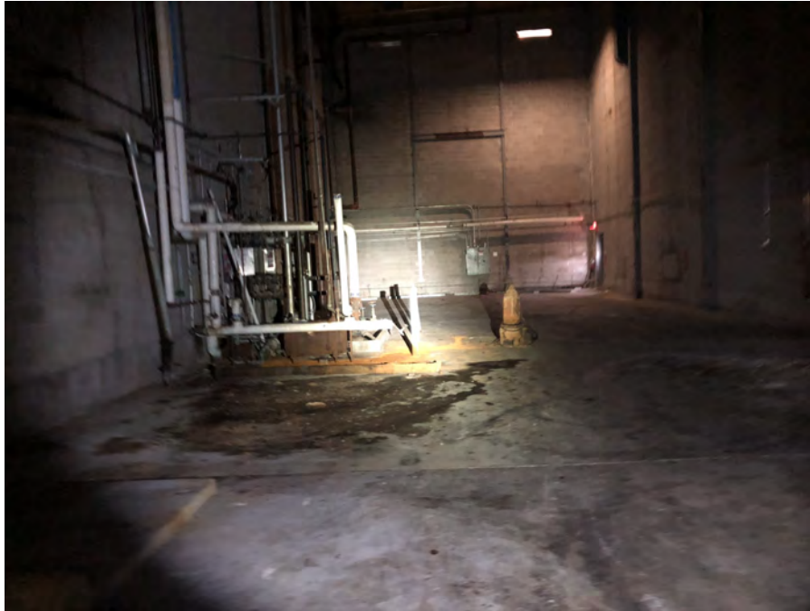
Photo 9: View of the dust collection area in Building 43. The sump pump is in the center-left section of the photograph.
