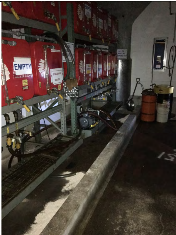
Photograph: 11 Former oil storage area in the basement of the facility. A rack of oil containers remained in place, but all level indicators appeared to be empty.
