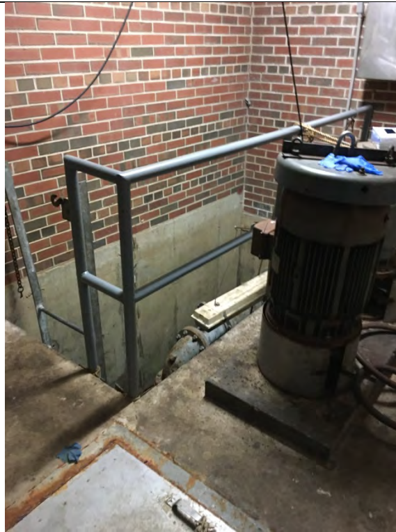
Photograph: 15 Sump room on ground floor historically tied into the on-Site water treatment plant. This particular sump was not currently collecting water, though the pump remained powered on.
