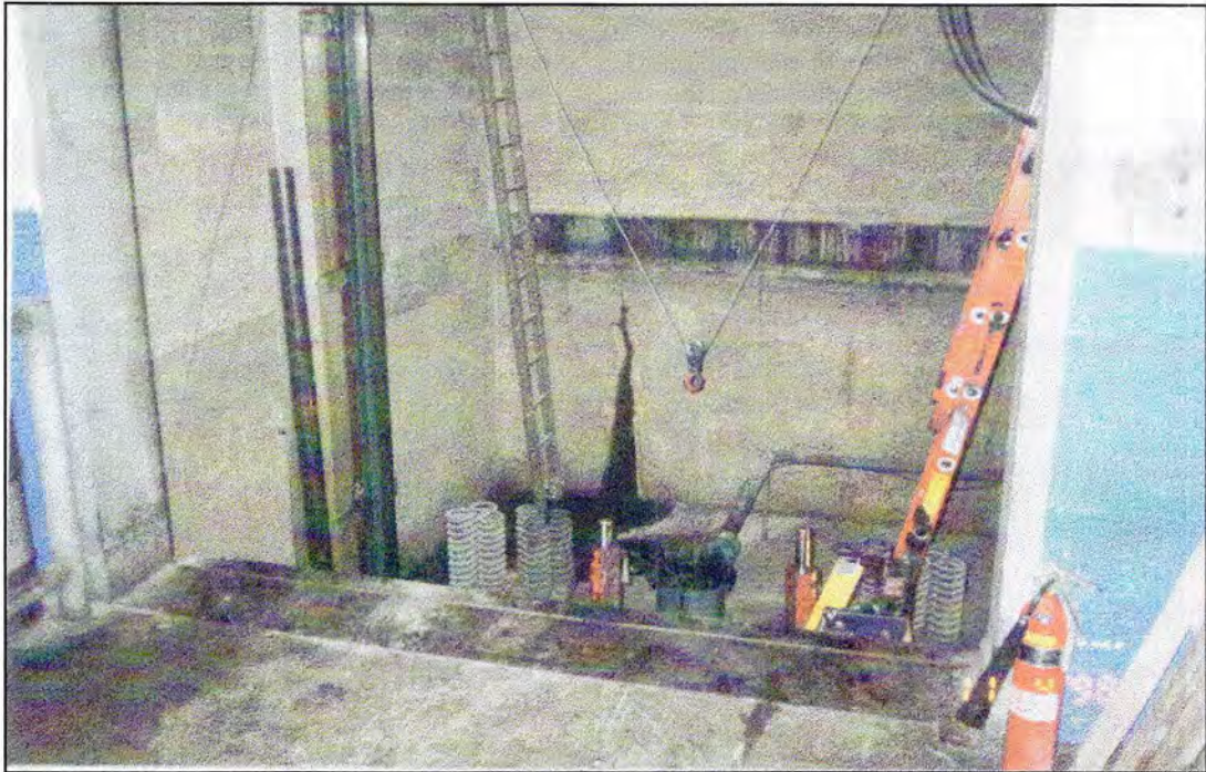
Photograph 1 Freight elevator room
