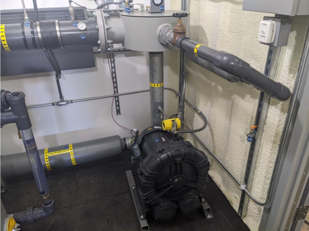
Figure 3: System Blower and piping
