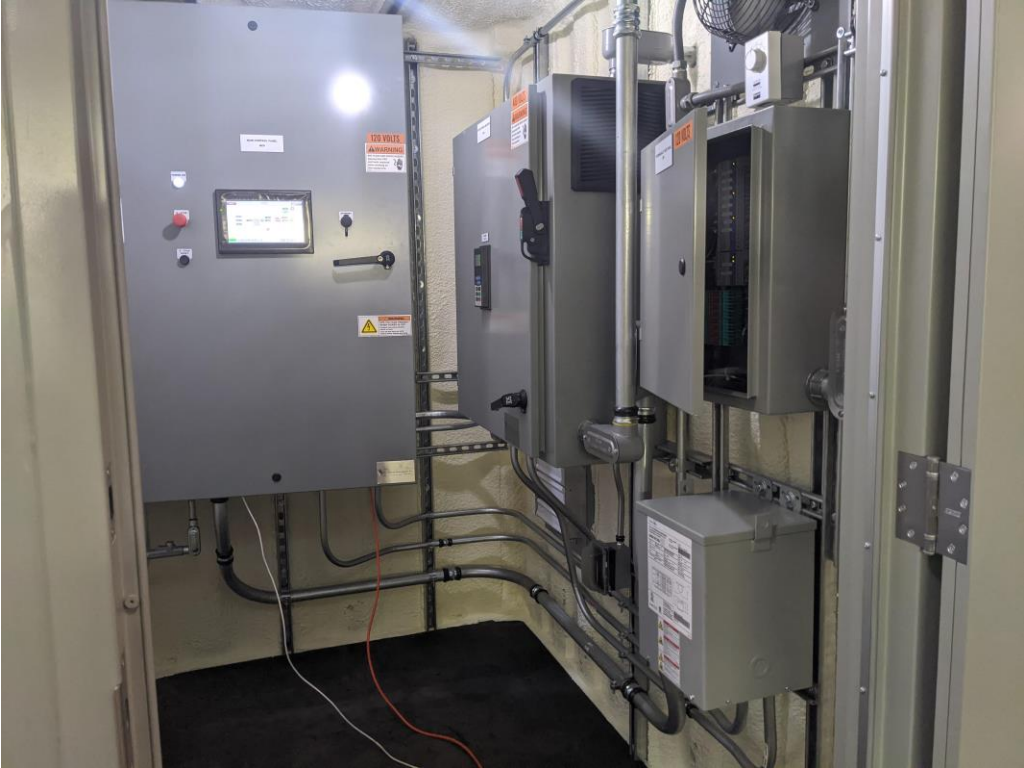
Figure 4: System Control Enclosure
