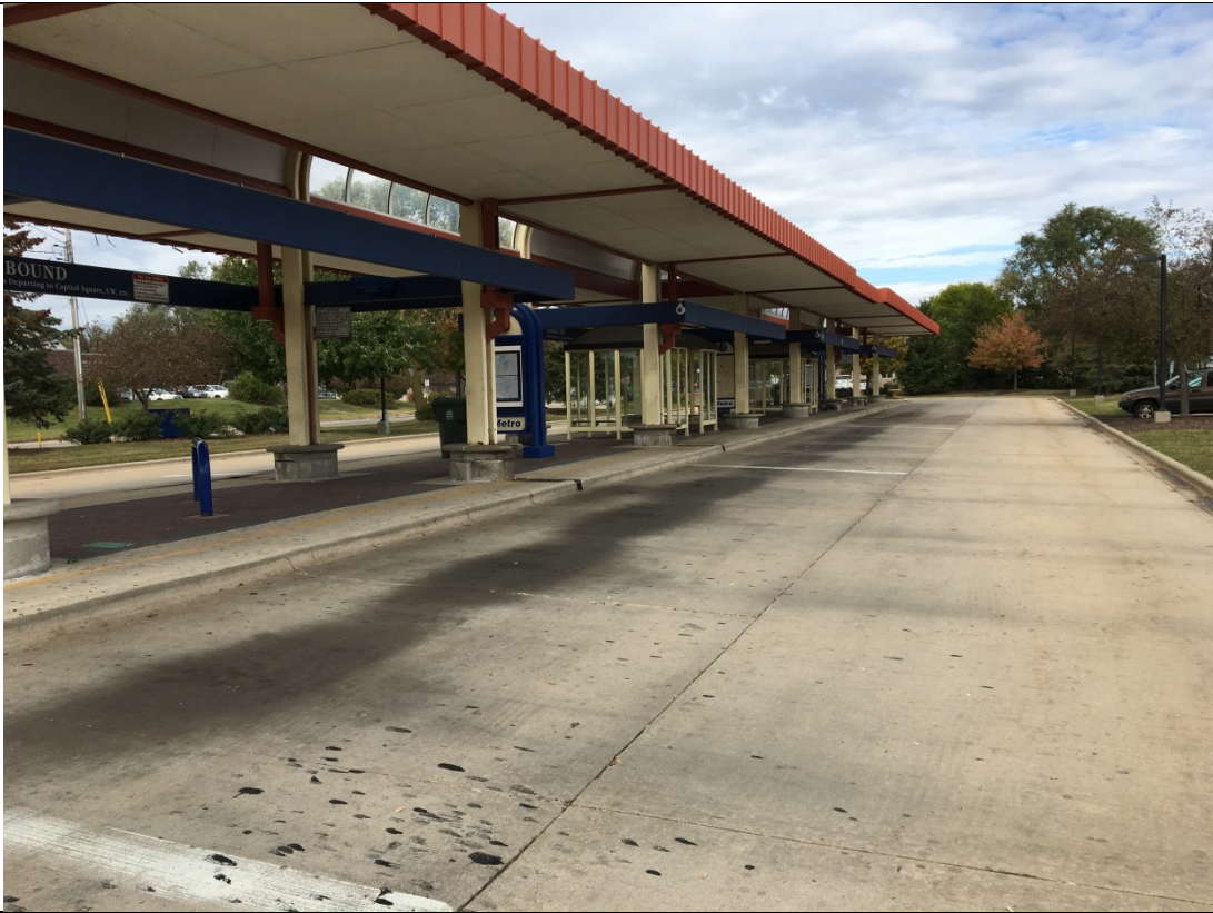
Photograph: 1 | Open-air, covered bus station located in the northeast portion of the Site.
