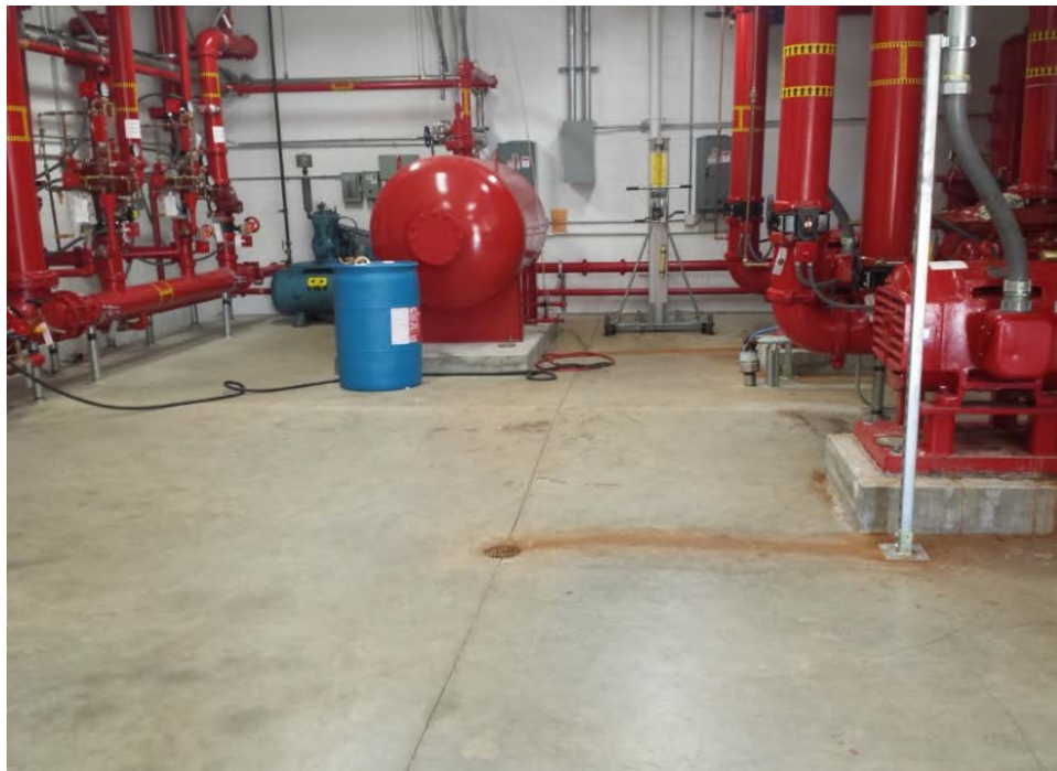
Photo 6: HEF storage (historically may have been AFFF storage) in the Mechanical Room of Hangar 406.
