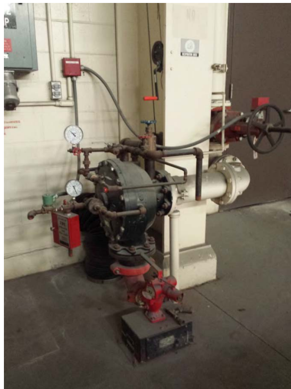
Photo 8: One of four fire suppression systems inside Hangar 414.
