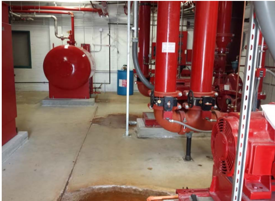
Photo 5: HEF storage (historically may have been AFFF storage) in the Mechanical Room of Hangar 400.
