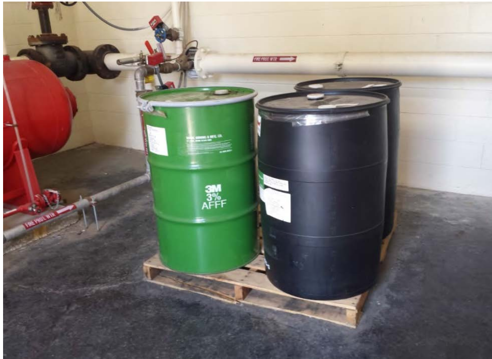
Photo 7: AFFF storage in the Mechanical Room of Hangar 414.
