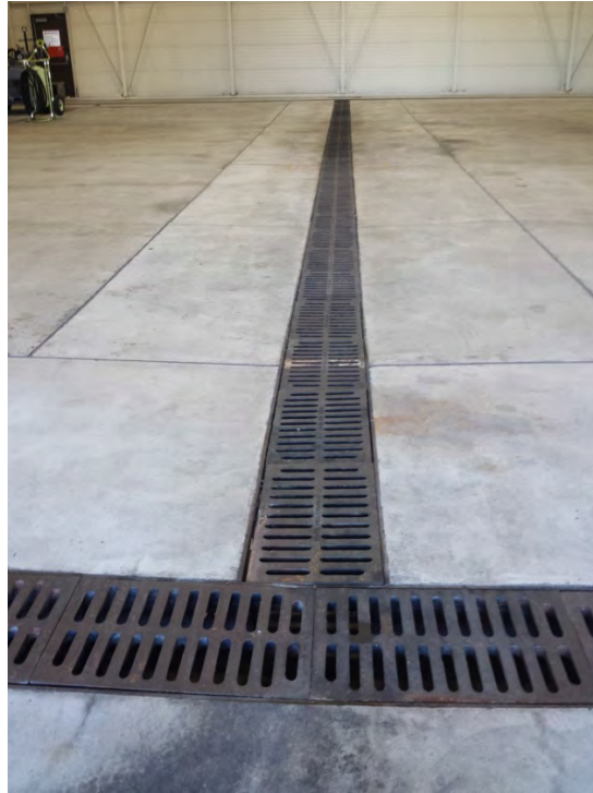
Photo 9: One of several trench drain inside Hangar 414.
