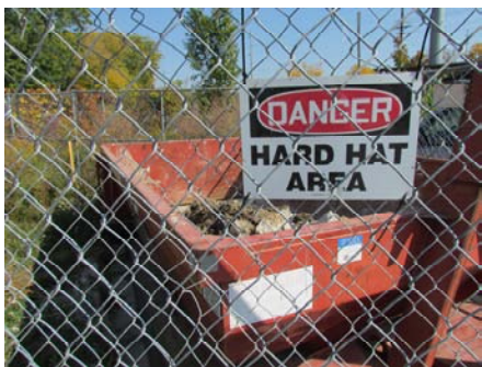
Dumpster full of soil excavated from the Goodman site. Where did it go? Was it contaminated? Should it have gone to a hazardous landfill? We'll never know.
