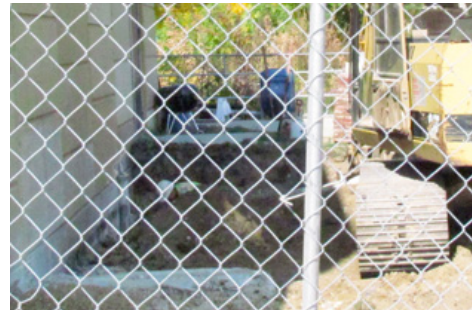
Worker (in hardhat, bending over) working below grade at Goodman Center (October 2012)
