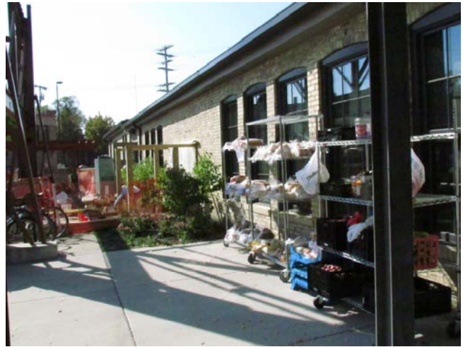
Food pantry bread and produce out during adjacent to the excavation site—free for the taking
